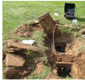
Portions of the tanks are uncovered
