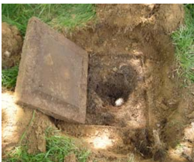
Root Clogged distribution box on a 4-year old system
