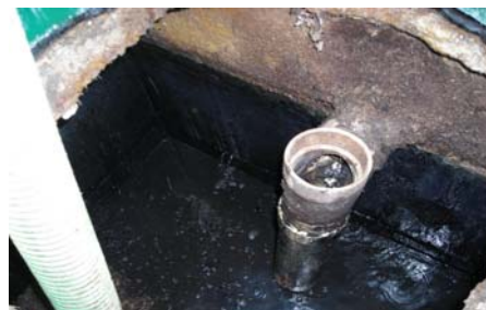
Septic Tank leaking at joint and riser on 15-year old system
